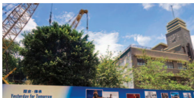
中電總辦事處已遭部分拆卸 Part of the CLP Headquarters building was demolished
