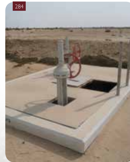
Valve pit in Ras Laffan
