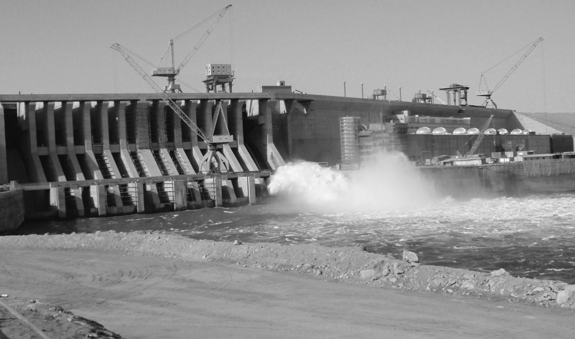
The Merowe Dam under construction on the fourth cataract, north of Khartoum, April 2009 Courtesy Donielle DeToy and Hussein Askary
