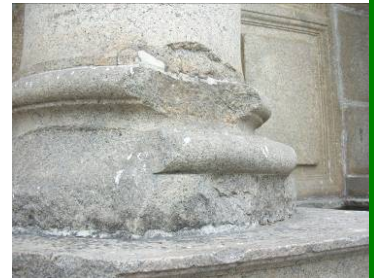
Photo F: Damaged pillars
