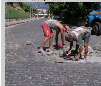
Fig. 3.4: Olinda, Brazil: Repair/replacement of damaged paving blocks is a part of the regular maintenance scheme of this World Heritage town.
