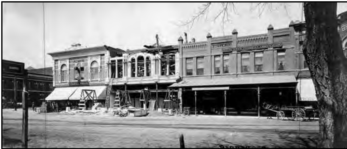
Figure 12. The Annex Block (1903), shown under construction, was erected by Lyman Robison and designed by Charles Rittenhouse. The F.L Smith Block is to the left and the Sulphide Building is to the right. SOURCE: Denver Public Library, Western History and Genealogy Department, Image Number X-6995.
