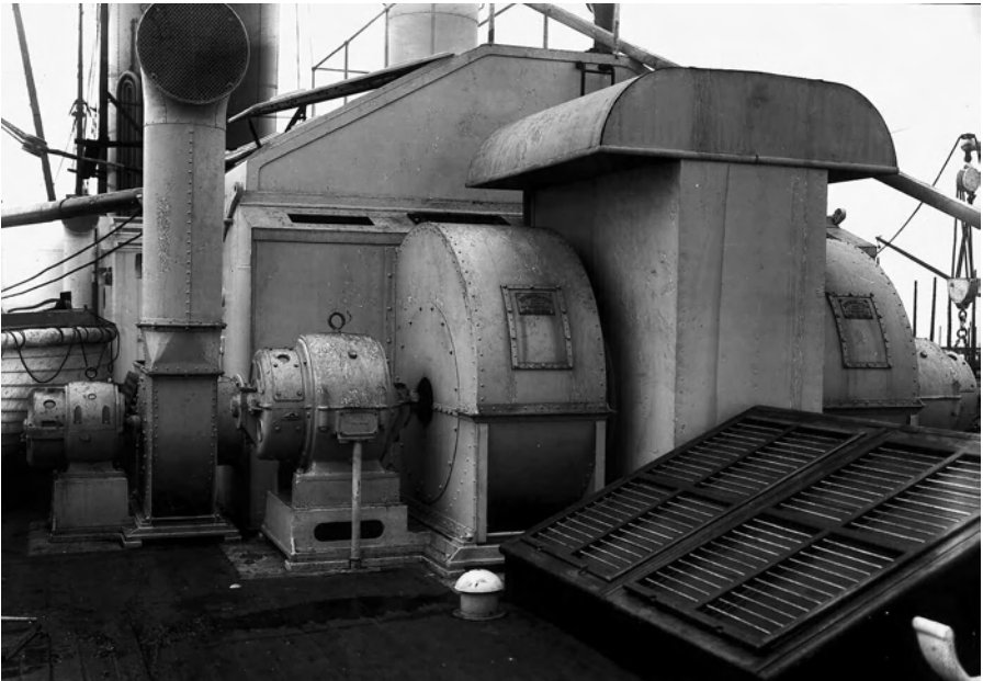
Fig. 7. 40 inch "Sirocco" Fans for Engine Room Ventilation.
