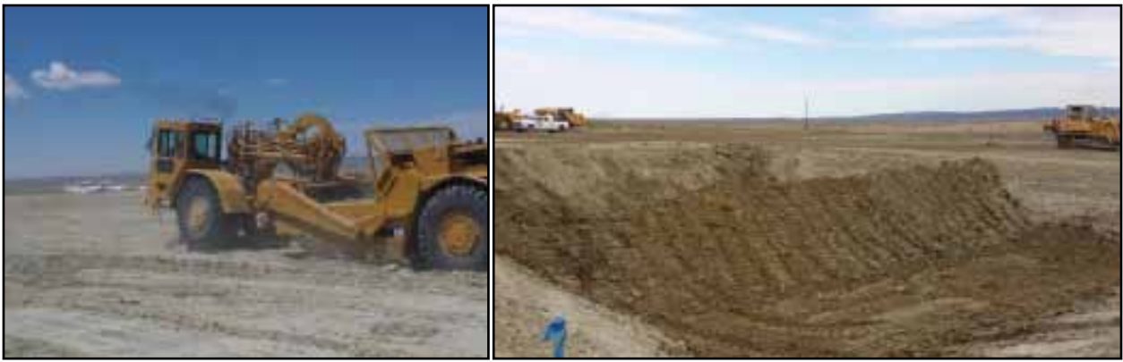
FIGURE 1. Left: belly-scraper removing bedrock on well pad in the Wind River Basin. Right: mud reserve pit on well pad in the Wind River Basin. Photography by R.J. Moses.
