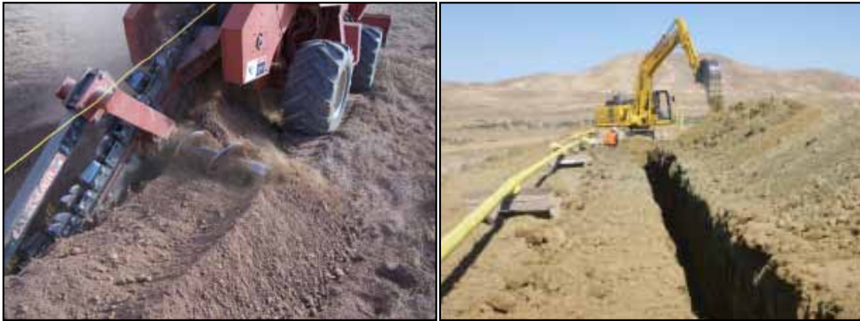
FIGURE 2. Left: Ditchwitch 7610 chain-style trencher with six inch cutting teeth. Electric trace wire (yellow) was installed into trench before piping was installed. Right: pipeline trenching using a tracked excavator. Spoils pile in right of image. Photography by R.J. Moses.
