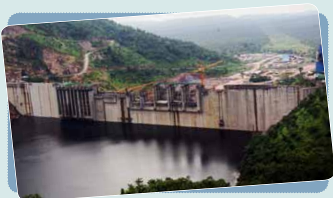
» Upstream View of the Bui Dam after impoundment as of July 2012 showing the three intakes (left) and the five spill gates (m) under construction
