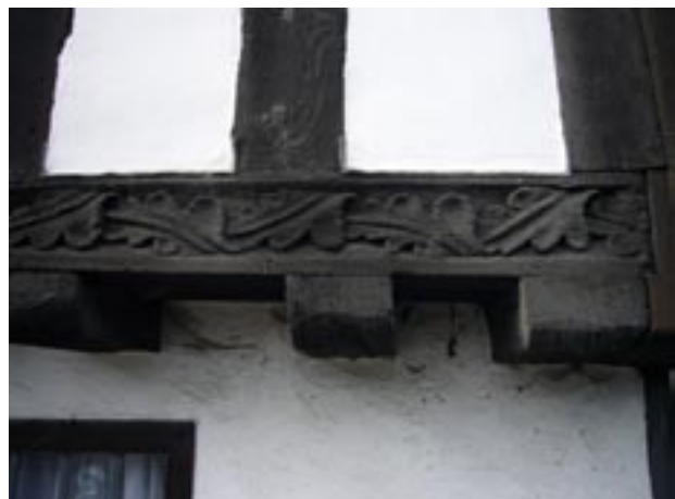
The Oaks, No. 82 High Street detail of carved bressumer
