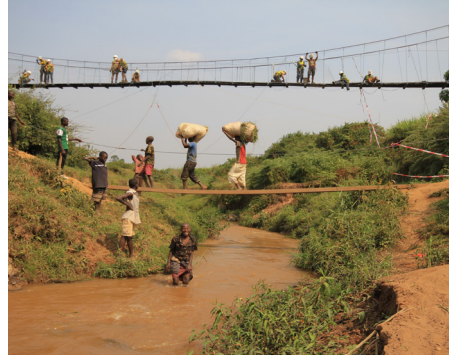
Log bridge and ford in use while the new Gaseke footbridge is built, Rwanda
