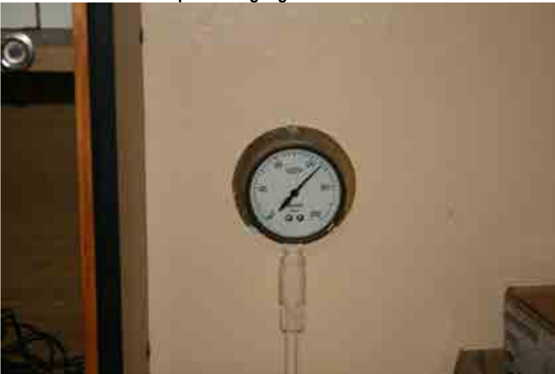
Downstairs town water pressure gauge
