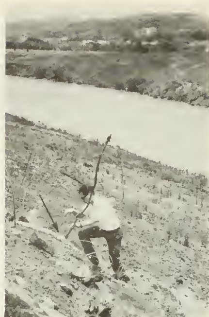
Gary Guazzo, soils mechanics engineer with the Panama Canal Engineering Division, probes a crack on the side of Hodges Hill.
