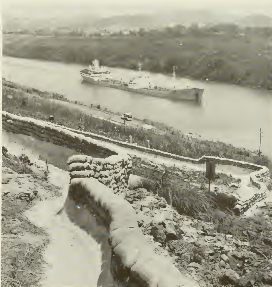
Concrete and sandbag lined walls and drainage ditches divert the storm runoff away from the slide area of Hodges Hill. A ship moves through the Gaillard Cut in an area where there might have been hazards to Canal traffic if preventive measures had not been taken.
