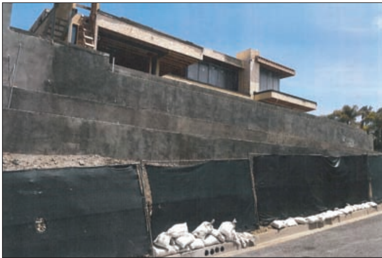
1251 SHADOW HILL WAY – The photo shows the close terracing used to inflate the size of the pad and the view impact.
