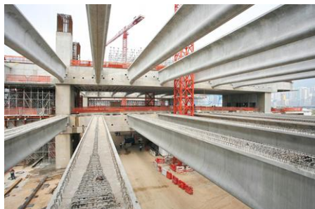
▲ The precast secondary beams of the first and second floors are supported on the primary box beams.
