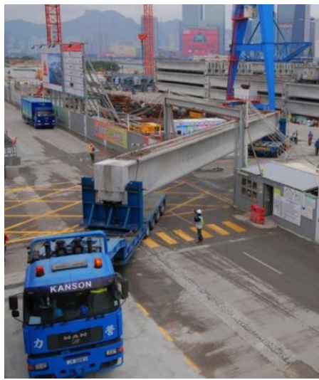
▲ A heavy-duty transporter moved the beams from the storage yard to the erection site.
