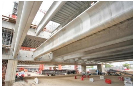
▲ The precast secondary beams of 1 st and 2 nd floor are spaced at 5.6m and support the ribbed precast slab.
