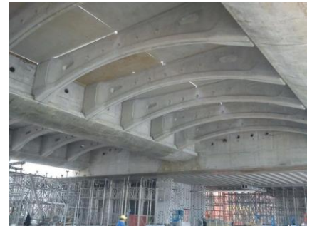
▲ View of the Roof Floor which is supporting the landscape deck. The framing is made up of post-tensioned primary and secondary box beams, with the later supporting the precast tertiary beams.
