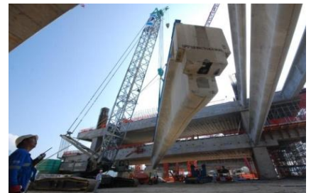
▲ A crawler crane was used to install the 31.5m-long and up to 125 ton heavy precast secondary beams onto bearings preinstalled along the halving joint of the primary box beams.
