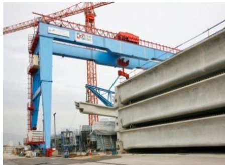
▲ The 240 precast secondary beams were cast and stored next to the site.
