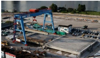
▲ View of the casting yard for the precast secondary beams at early stages. The casting yard had 5 moulds for casting, one bay for curing and stressing and 2 bays for storage of the beams.
