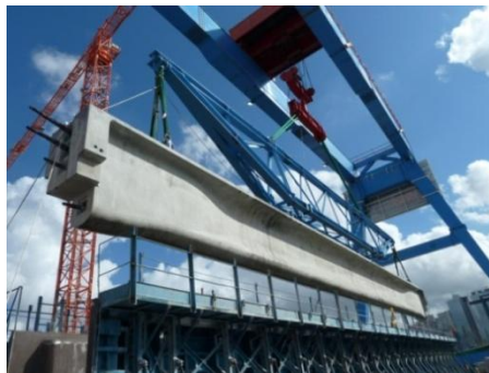
▲ A 150t-capacity portal gantry handled the precast secondary beams at the casting yard.
