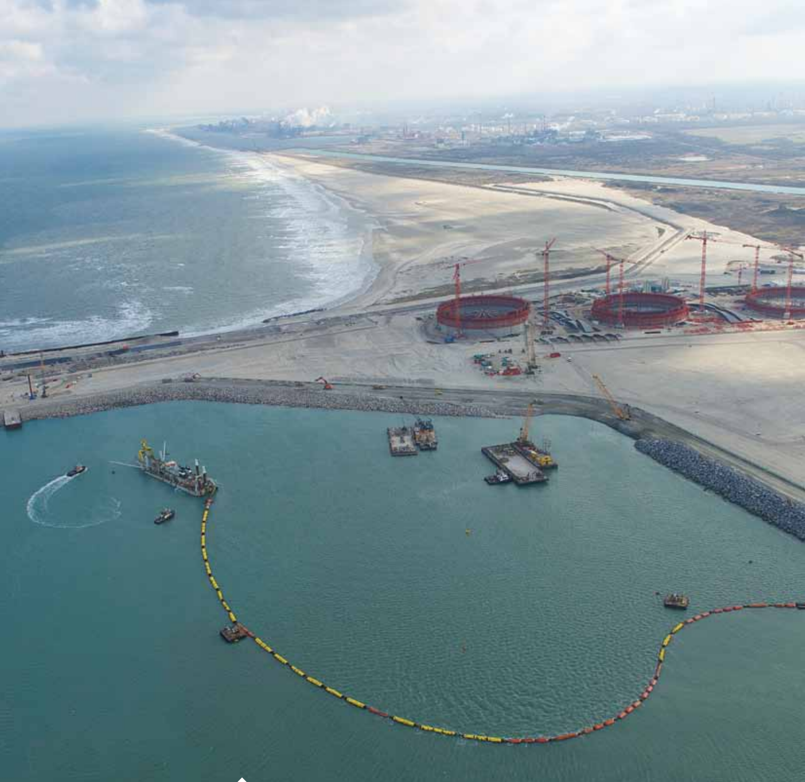
Construction of port facilities for a future liquefied natural gas (LNG) terminal in the outer Western Port of Dunkirk (France)
