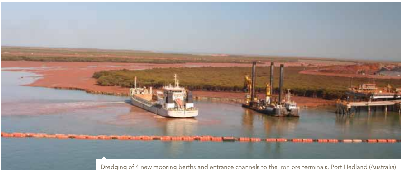
Dredging of 4 new mooring berths and entrance channels to the iron ore terminals, Port Hedland (Australia)
