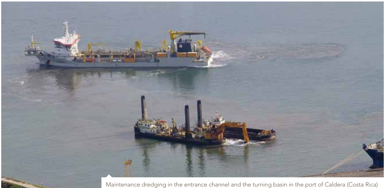
Maintenance dredging in the entrance channel and the turning basin in the port of Caldera (Costa Rica)
