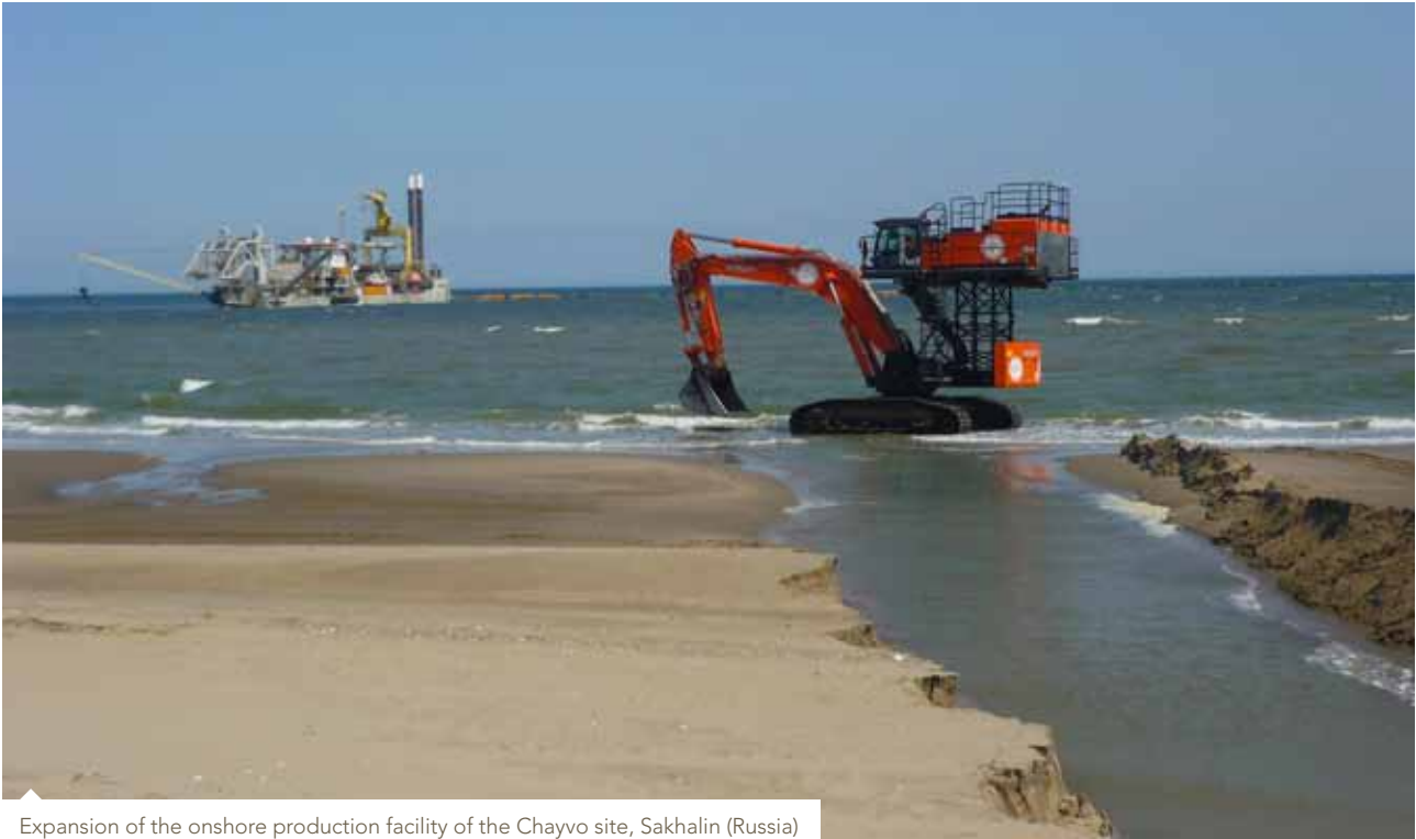
Expansion of the onshore production facility of the Chayvo site, Sakhalin (Russia)
