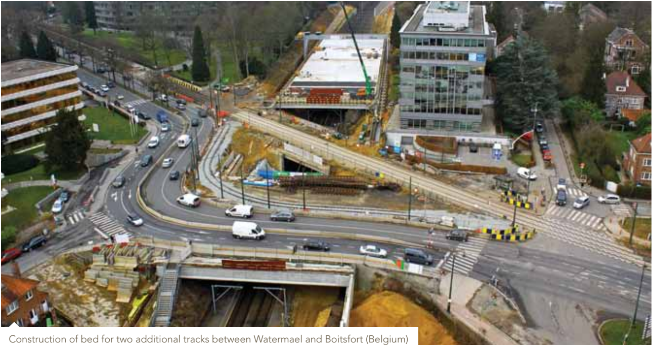
Construction of bed for two additional tracks between Watermael and Boitsfort (Belgium)
