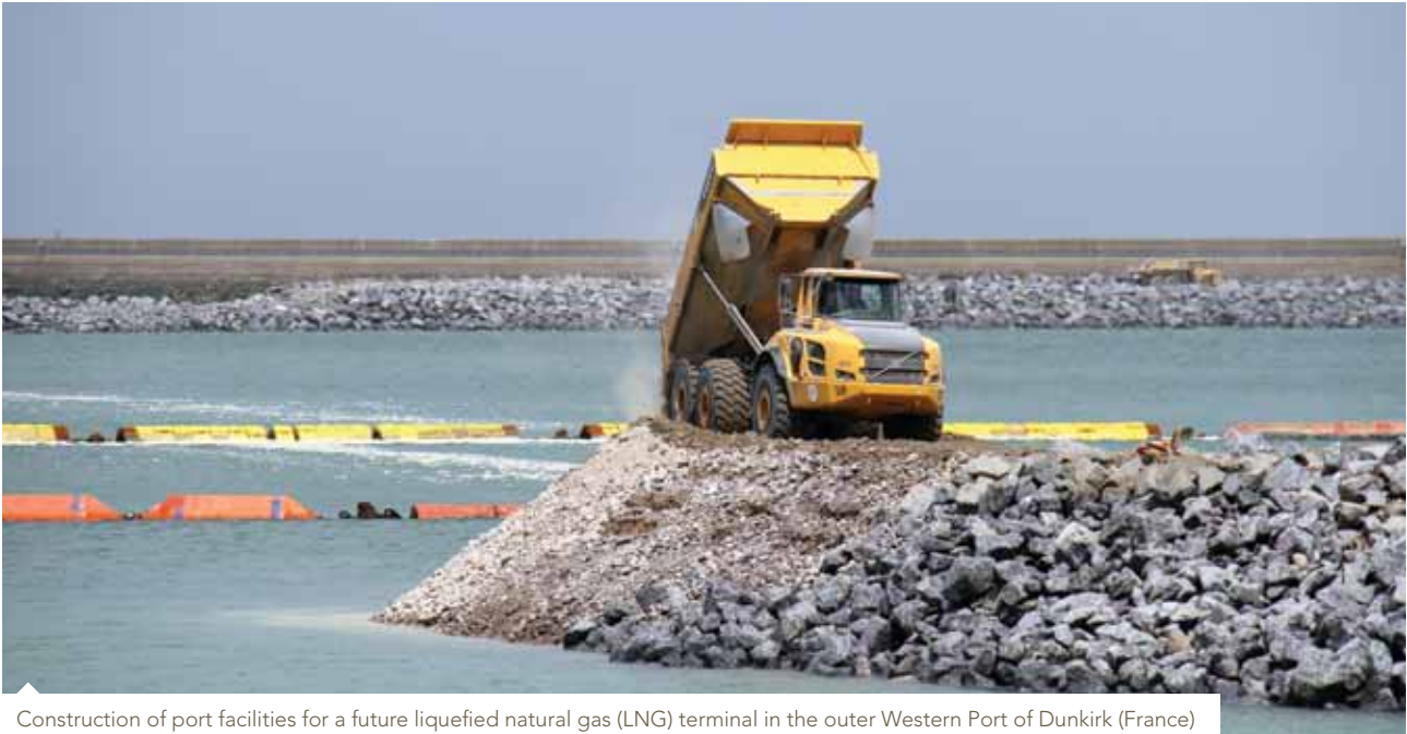
Construction of port facilities for a future liquefied natural gas (LNG) terminal in the outer Western Port of Dunkirk (France)
