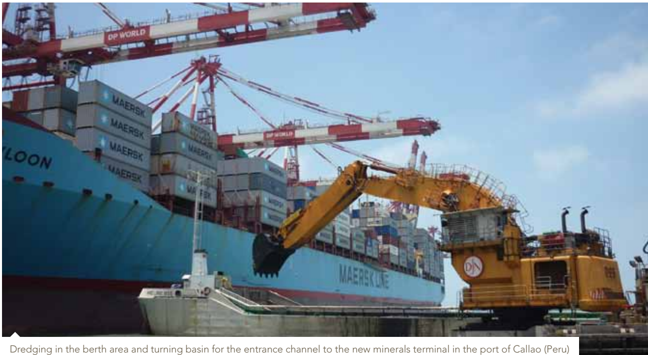
Dredging in the berth area and turning basin for the entrance channel to the new minerals terminal in the port of Callao (Peru)
