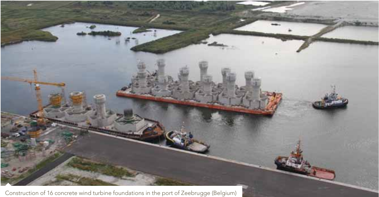
Construction of 16 concrete wind turbine foundations in the port of Zeebrugge (Belgium)
