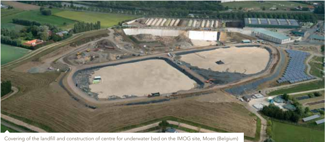
Covering of the landfill and construction of centre for underwater bed on the IMOG site, Moen (Belgium)
