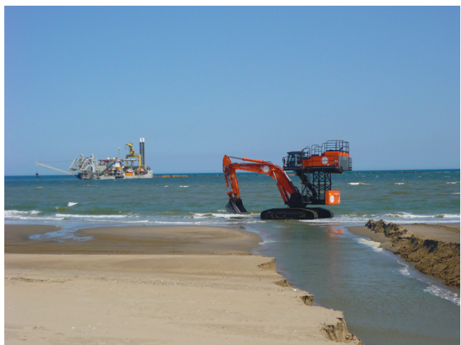
Figure 7. Jan De Nul Group's cutter suction dredger Fernão de Magalhães and Starfish I executing trenching works.
