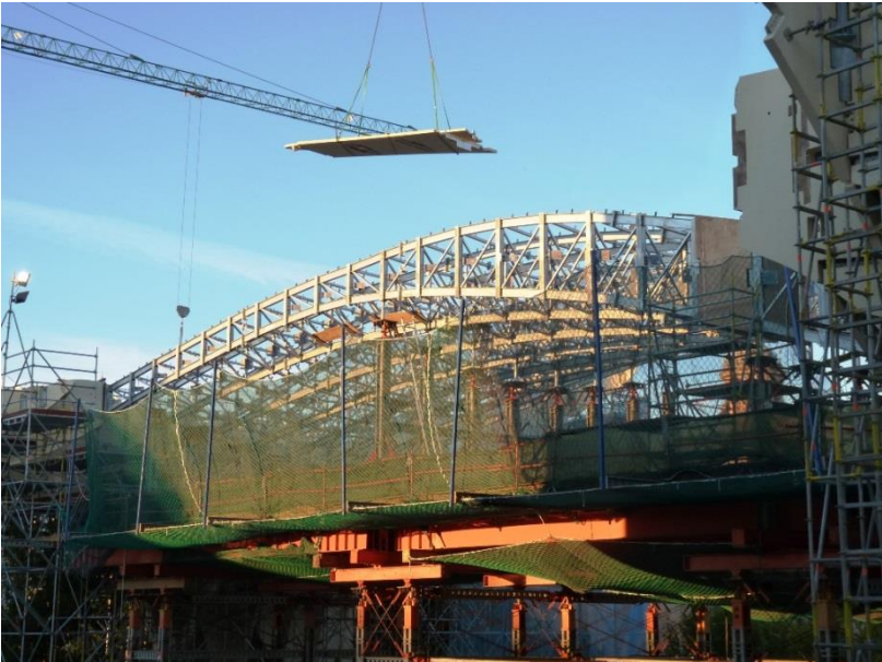
Fig. 5 Steel load-bearing platform of the restaurant and cafe area (above) Steel structure crossing the main road under traffic (below)
