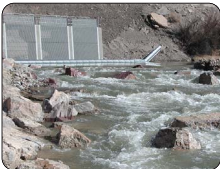
Construction of a weir wall to prevent fish from entering the Hogback Irrigation Canal will begin in 2010. Fish passages are being considered at the Arizona Public Service Company Weir and the Fruitland Diversion Dam.
