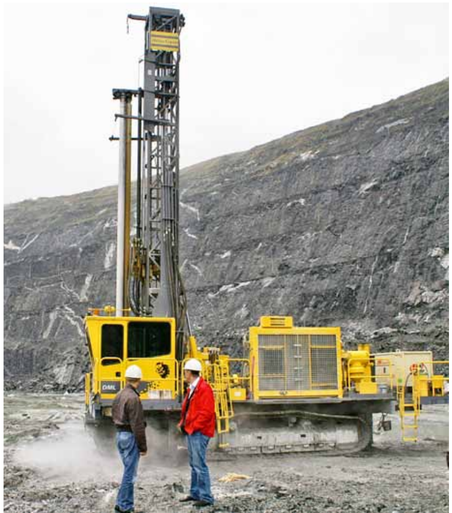
Contractor Technobur has four Atlas Copco Drilling Solutions DML rigs working for Kovdorsky GOK. Three are low pressure (LP) rigs for rotary drilling, and one is a high pressure (HP) rig for DTH drilling or rotary drilling.
