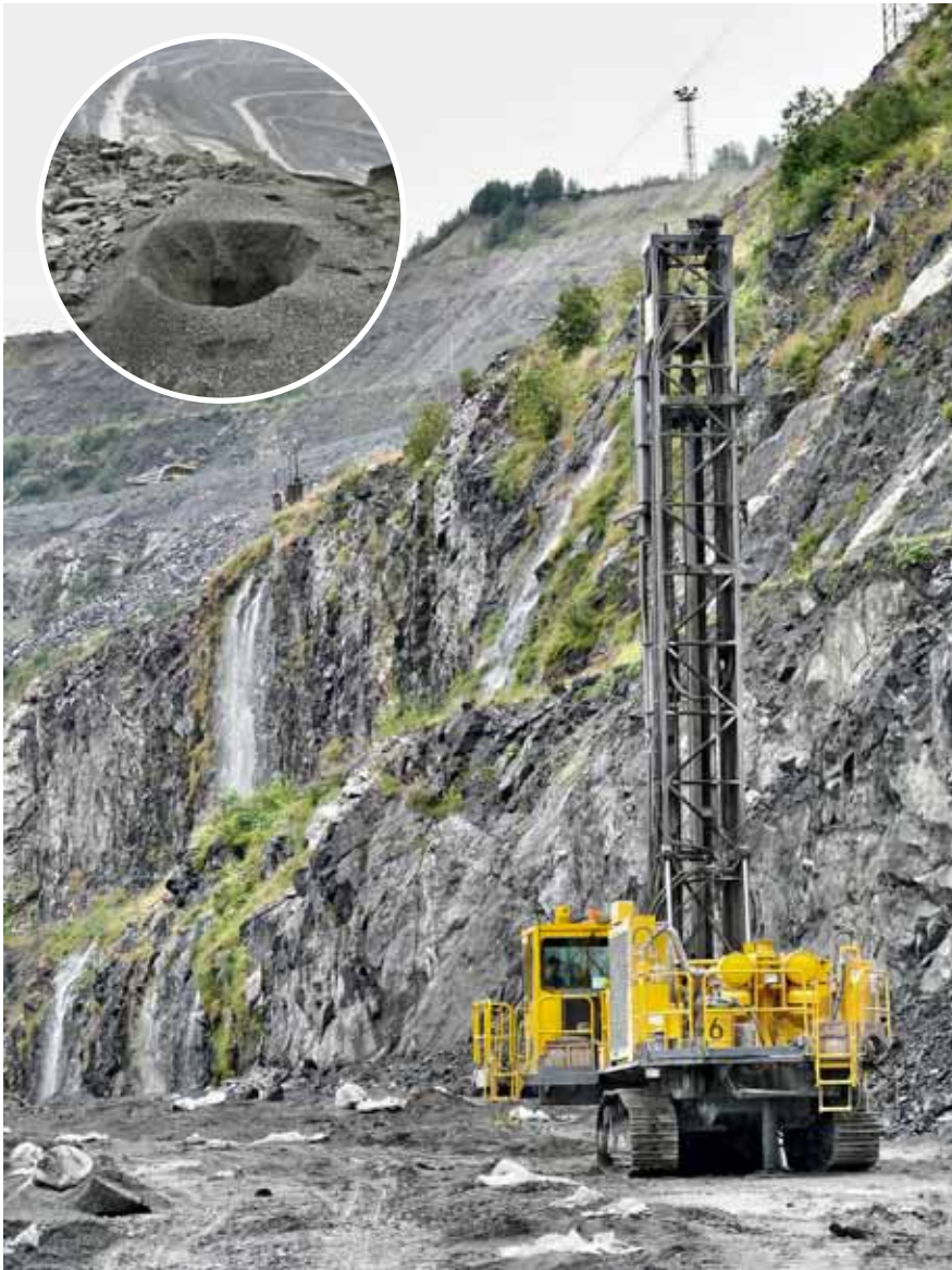
A major player in Kovdovsky's Super Deep Mining programme: Atlas Copco's DM45 HP (high pressure) rig on the pit's upper, 12 m high benches.
