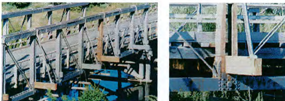
Figure D A general view of a deBurgh composite truss and a closer view of a pinned joint in the bottom steel member with new replacement timber.
