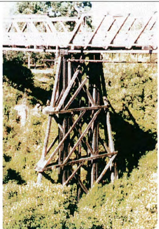
Upper portion of the 64-foot trestle, the deck is 92 feet above the water.
