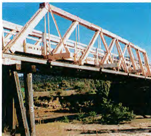
Figure E A typical composite Dare truss of the Howe type with timber diagonals and riveted steel bottom chord.
