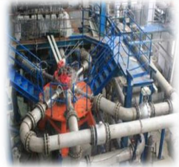
Facility for hydro-simulation
