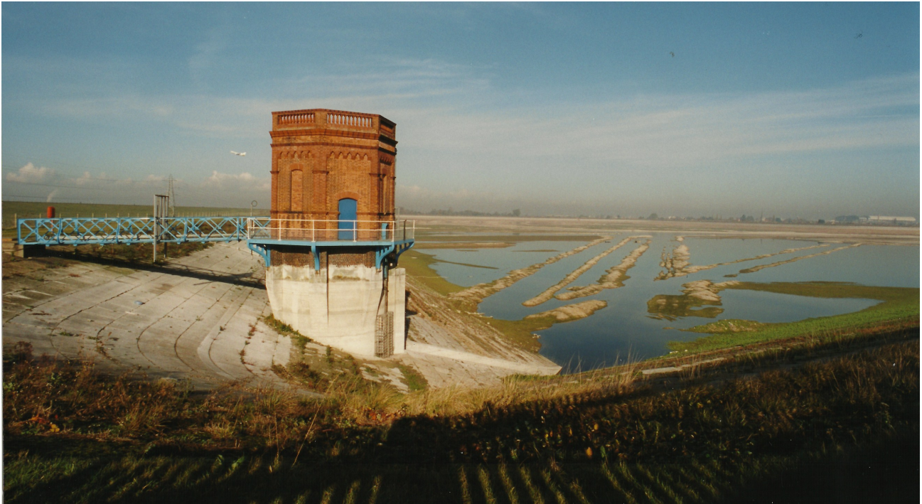
One of the twin, back-to-back Staines reservoirs of the West Middlesex Water Company, photographed with the water down in 1998.
