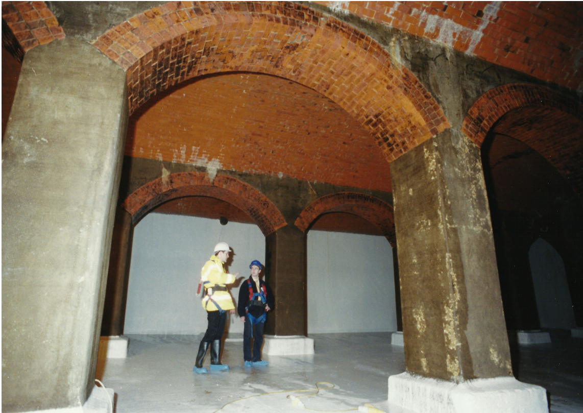
Interior of the Victoria Reservoir, Farnham, a typical covered reservoir. The photograph was taken during cleaning and renovation in 1999, 100 years after the reservoir was opened.
