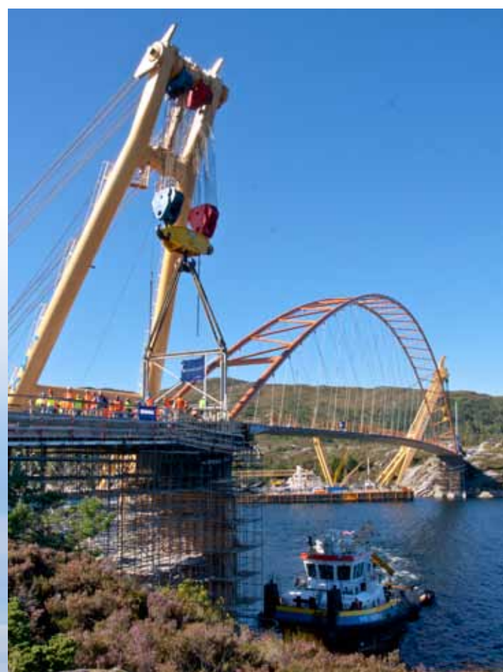
'Taklift 4' and 'Taklift 7' installing the 220 m long bridge section in dual lift.
