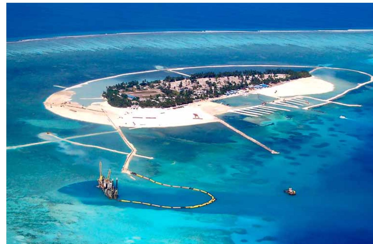
Boskalis restored the island of Vilufushi, which was devastated by the tsunami in 2004. The island was extended threefold, raised and provided with coastal defenses.
