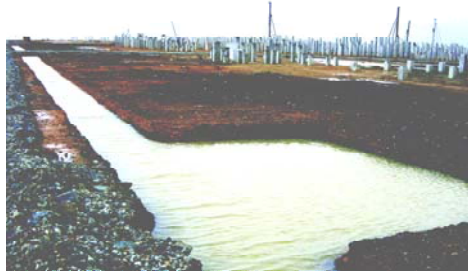
Drainage system and sedimentation basins to catch rain water run-off
