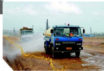
Watering trucks work around the clock to damp down dust from site
