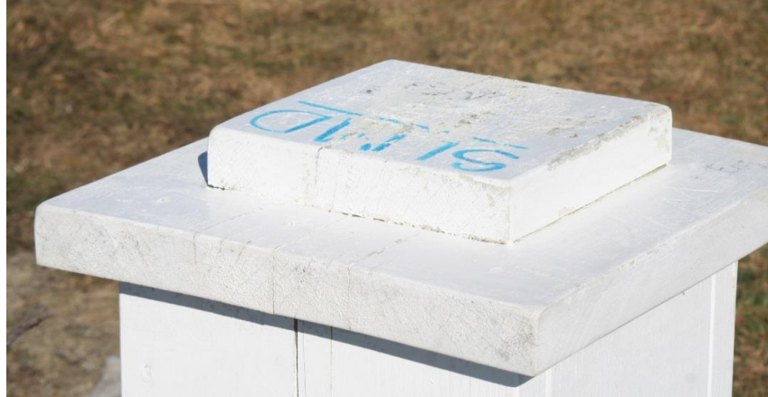
Figure 21: Graffiti on one of the pillars. Other graffiti has noticeably been painted over.
