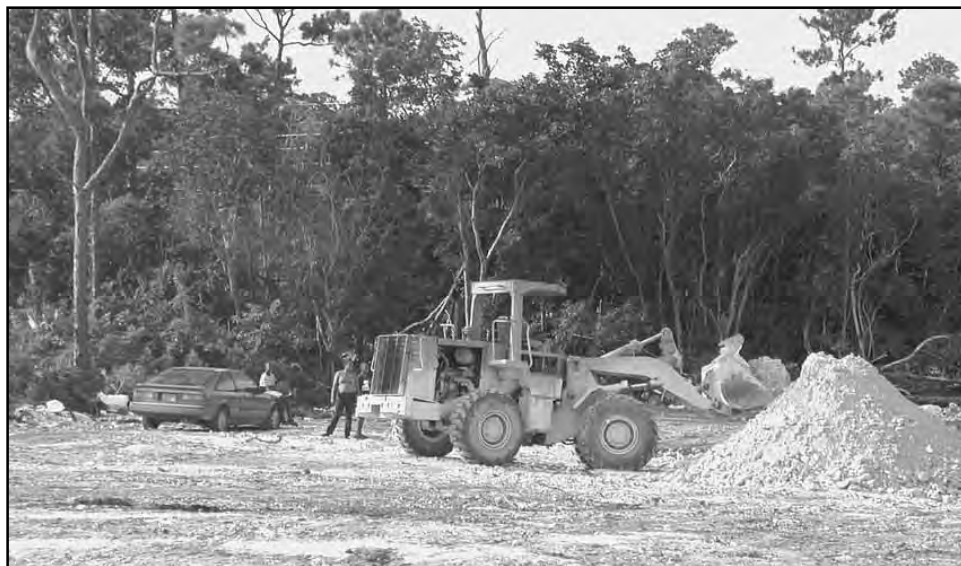
This is the first lot to be cleared in Central Pines Estates belonging to Carol and Scott Davis. Mr. Davis works for Bahamas Hot Mix and hopes to begin construction soon. Many applicants are getting their paper work prepared and loans arranged. The government subdivision offers generous sized lots with all utilities in place for a reasonable cost.
