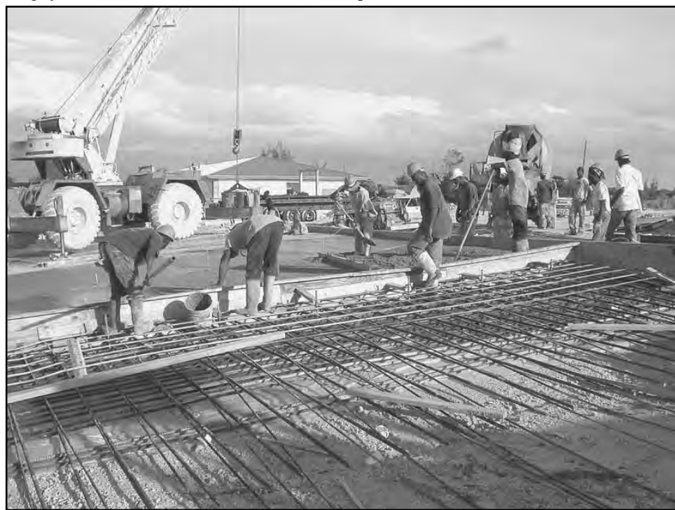
The concrete apron around the entire dock area is under construction. Two hundred feet is complete in front of the domestic warehouse and is being used by freight boats. The interior area of the space will be paved with a chip-and-seal surface. The project entails moving the main road back and constructing a new road connecting the dock with Crockett Drive and S. C. Bootle Highway. All the road work is well underway.
