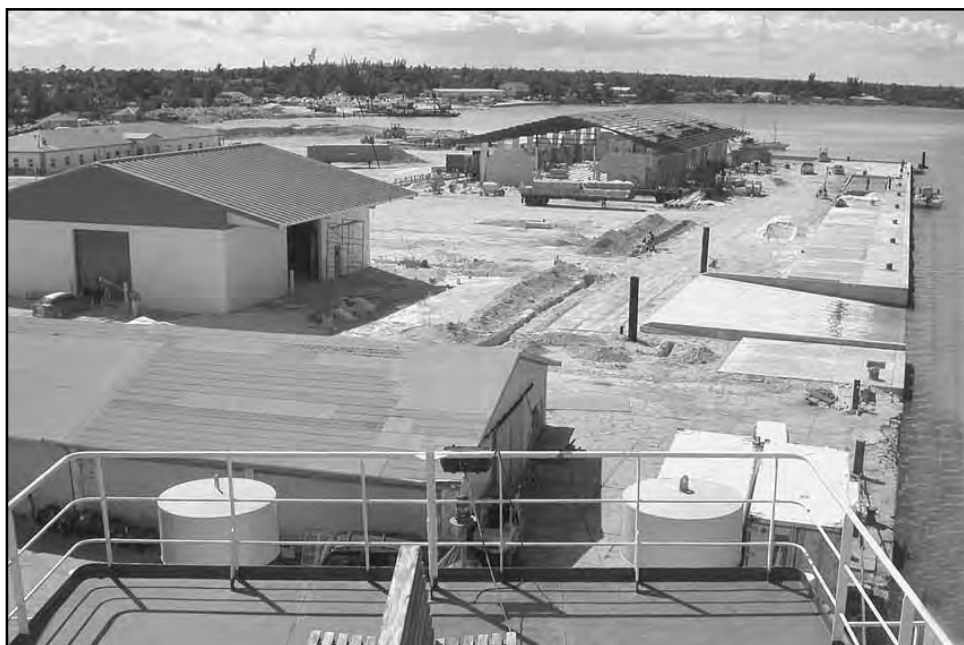
Construction of the new freight dock in Marsh Harbour is progressing rapidly. The domestic warehouse shown on the left is now complete and is being used by Customs and the freight companies until the project is complete. The large building pictured in the far center is the international warehouse under construction. The concrete apron around the entire dock area is being poured. On the right is one of the ro-ro ramps which accommodates the offloading of cargo from boats with either a bow or stern ramp.
