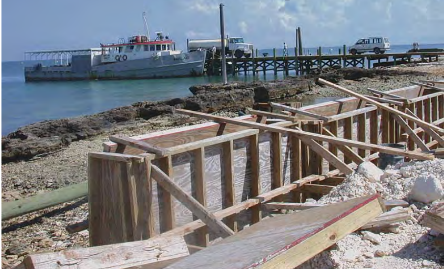
Cooper's Town, heavily damaged by Hurricane Floyd in September 1999, suffered the loss of their sea wall and public dock. The dock is now finished and the seawall is nearing completion. The sea wall, several thousand feet in length, is built in sections. A wide concrete sidewalk is added behind the wall, giving additional protection.
