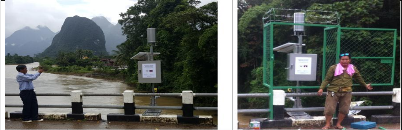
Automatic Water Level Station including Raingauge at Vang Pho Bridge
