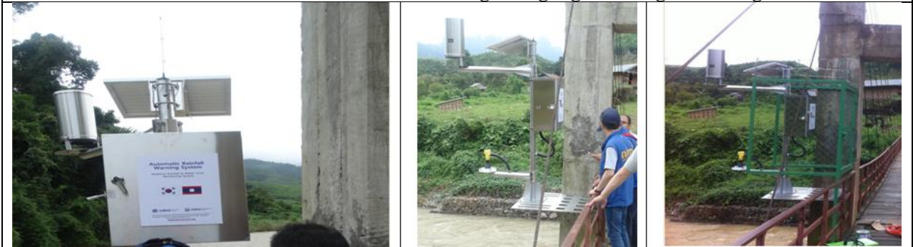
Automatic Flash Flood Early Warning Post at Ban Muang Song
