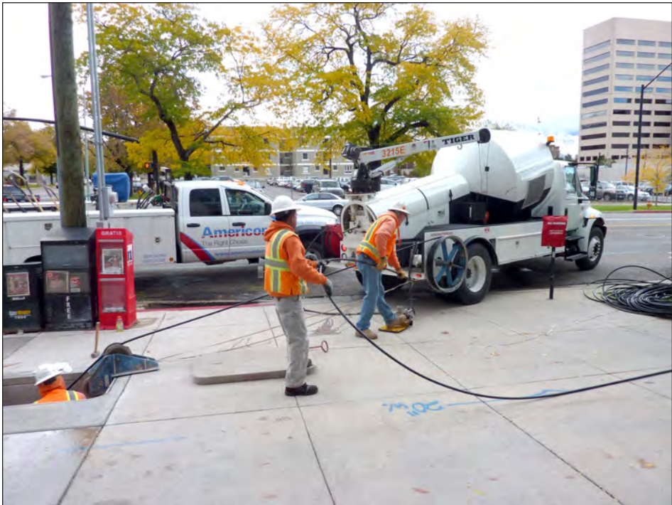
UDOT has woven broadband into rights-of-way along state roads.
