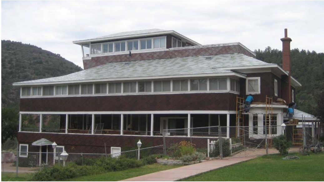
The "Notice to Proceed with Construction" was issued Monday, May 18, 2009, for "Structural Repairs and Roof Replacement" at the Historic Tonto Lodge. New glu-lam beams and support posts have been added under the dining room and lobby floors.
