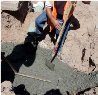
Construction work continued at McFarland. Pictured here, concrete bases for the storm drainage collectors in progress.
