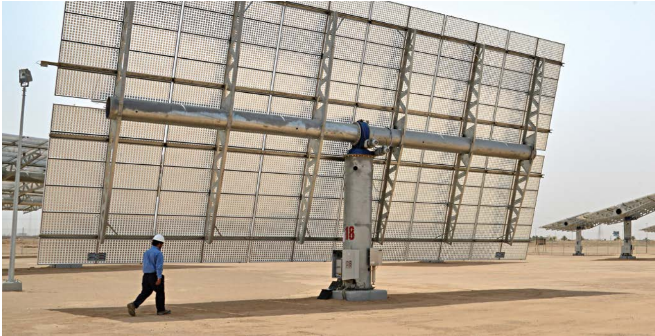
The 1 megawatt concentrated photovoltaic system at our Tabuk Bulk Plant is the first such utility-scale plant in the Middle East.
