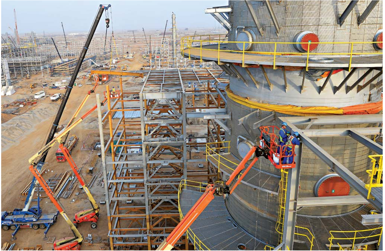
Our refinery under construction in Jazan will form the industrial heart of the greater Jazan Economic City, helping drive sustainable economic growth in the region.
