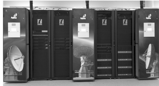
Fig. 2 View of the high-performance computing cluster based on the hybrid blade servers.
