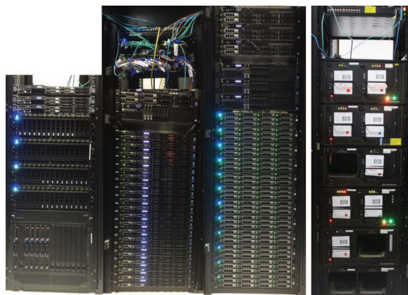
Fig. 2 DiFX cluster system and Mark 5A/B units.
