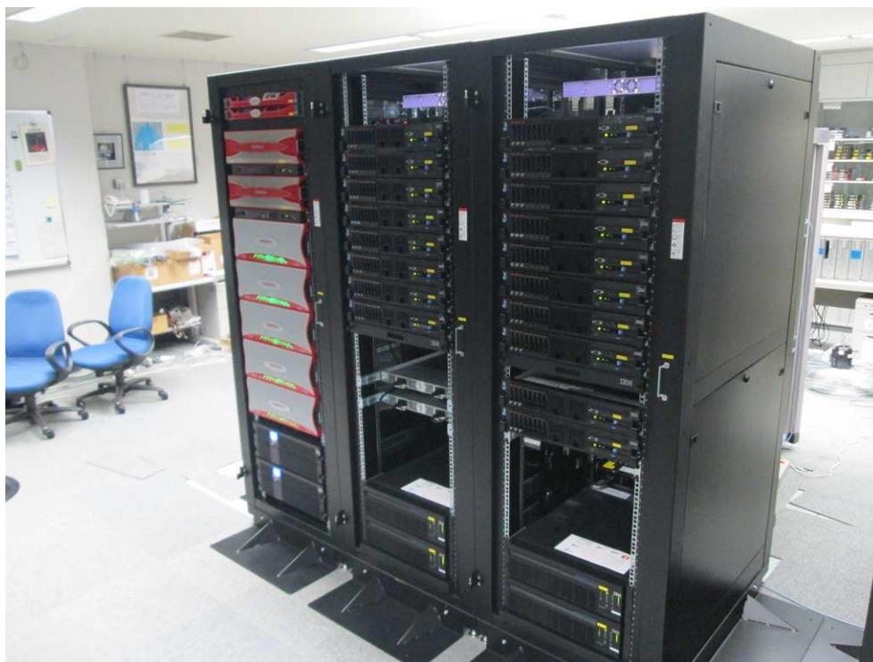
Fig. 1 View of the data processing servers and storage system at the Tsukuba VLBI Correlator.
