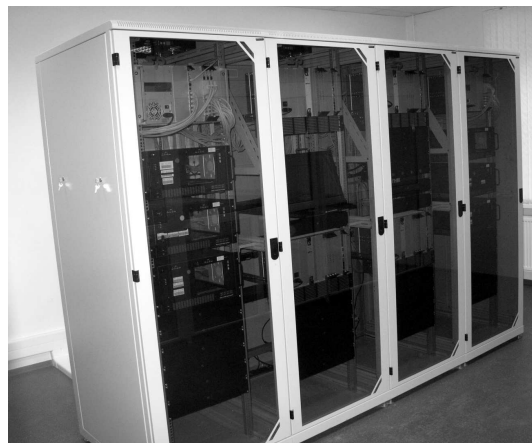
Fig. 1 View of the six-station ARC correlator, showing four racks containing (left to right) signal distribution and synchronization system (SDSS) and three Mark 5B playback units, two correlator crates and a KVM, three correlator crates, and one more cabinet with an SDSS and three Mark 5B playback units.
