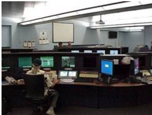
DSCC Signal Processing Center (SPC) located at the DSN complex
