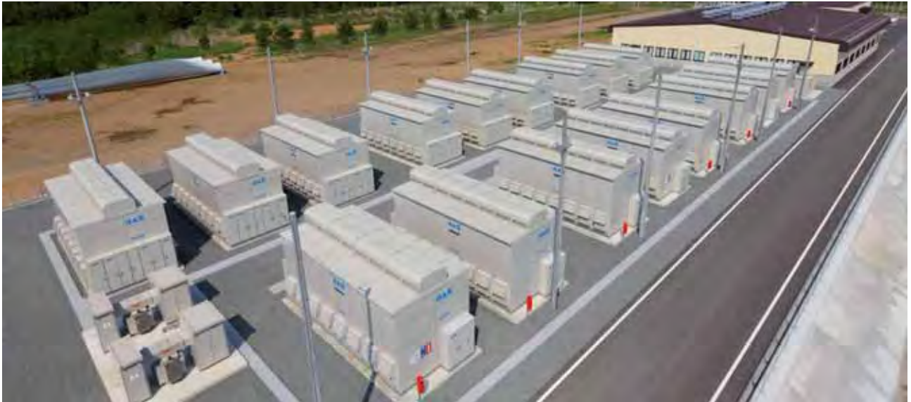
Figure 3-10 | NaS battery units – 34 MW (Japan Wind Development Co.)
