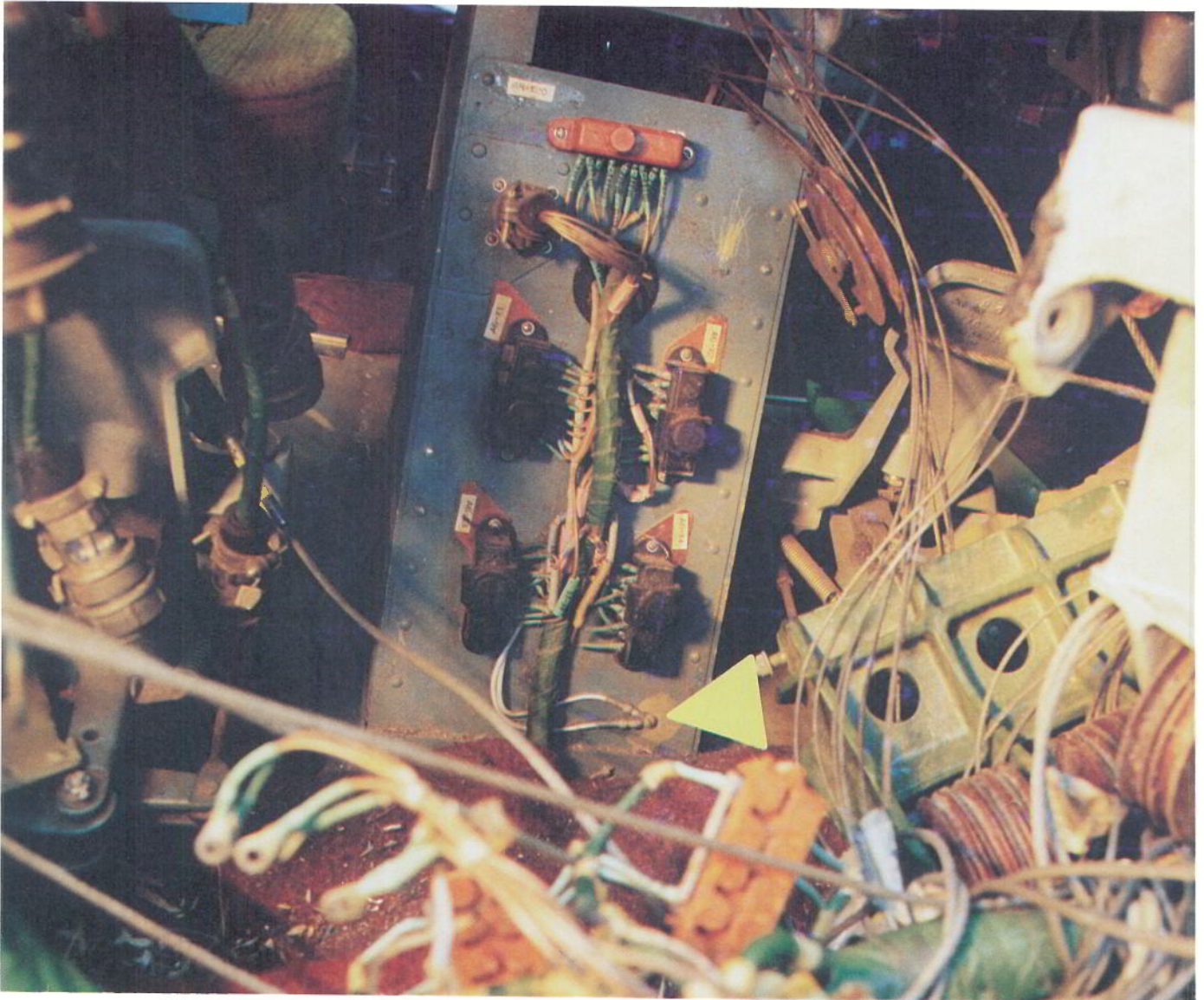
Figure 3 Showing terminal block A6X1 with loose earthing screw arrowed
