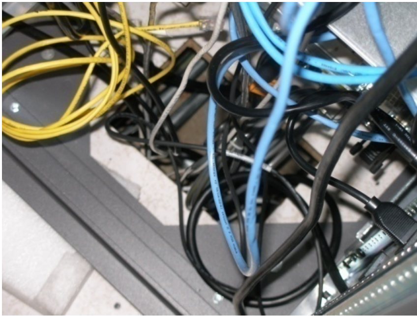
Unsealed cable penetration (inside rack)
