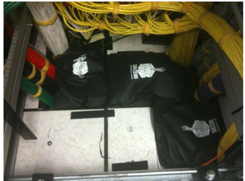
Sealed cable penetration
