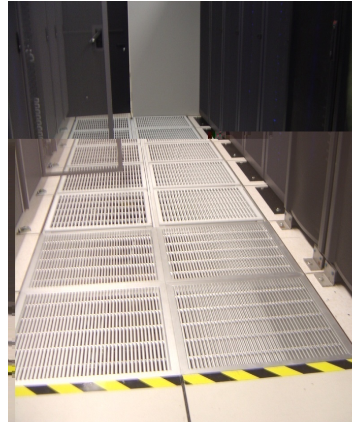
High-flow tiles reduced air pressure
