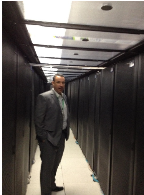
APC Hot Aisle Containment (with in-row cooling)
