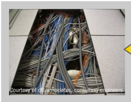
Congested Floor & Ceiling Cavities
