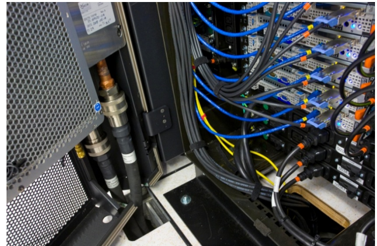
Liquid Cooling Connections
