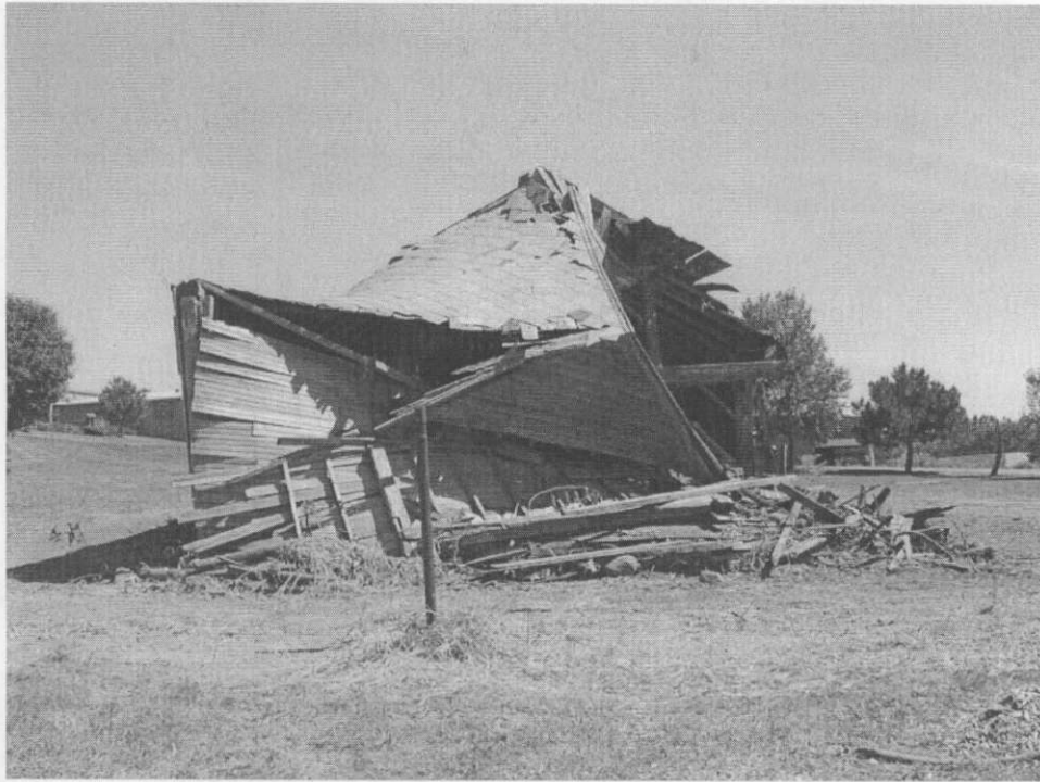
Picture 3. Exterior West Wall. This part of the roof collapsed several years ago.
