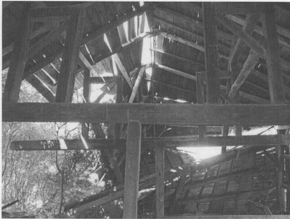
Picture 7. Interior West Wall. This part of the barn roof collapsed several years ago.
