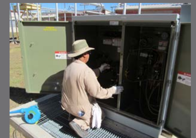
Frankie Diaz at Pantex cleans the interior of a de-energized 12,470/480-volt transformer.
