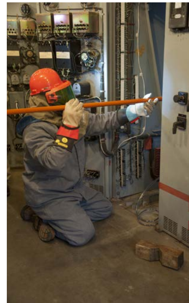
Y-12's Ed Crowder checks for absence of voltage in a 4,160-volt switchgear using the appropriate electrical personal protective equipment.
