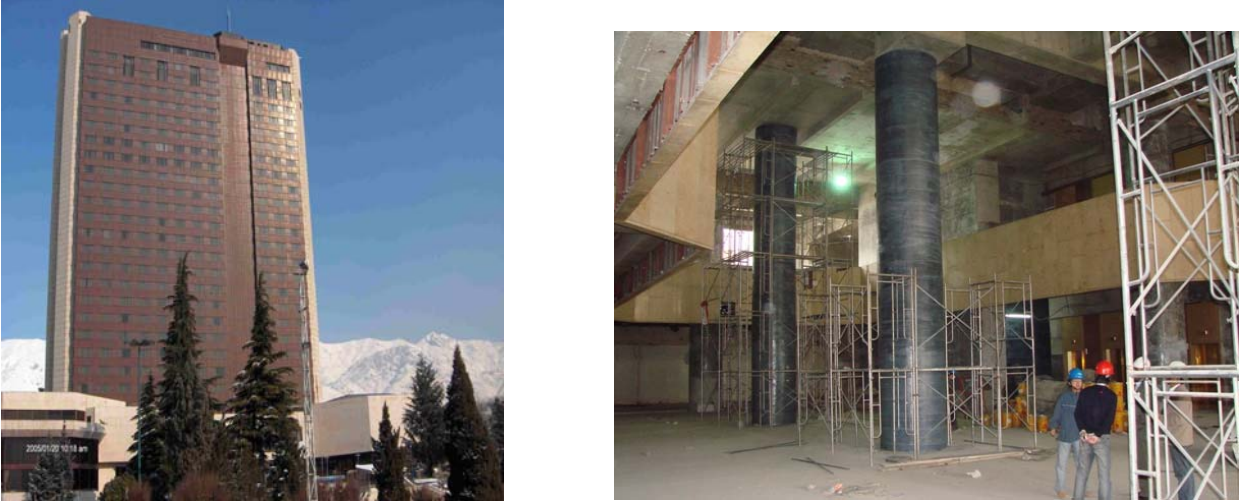
Fig. 1. Left: Parsian Azadi Hotel in the northern part of Tehran, Iran: main tower, south elevation, Right: Columns at the hotel lobby with a diameter of 1.5 m wrapped with CFRP
