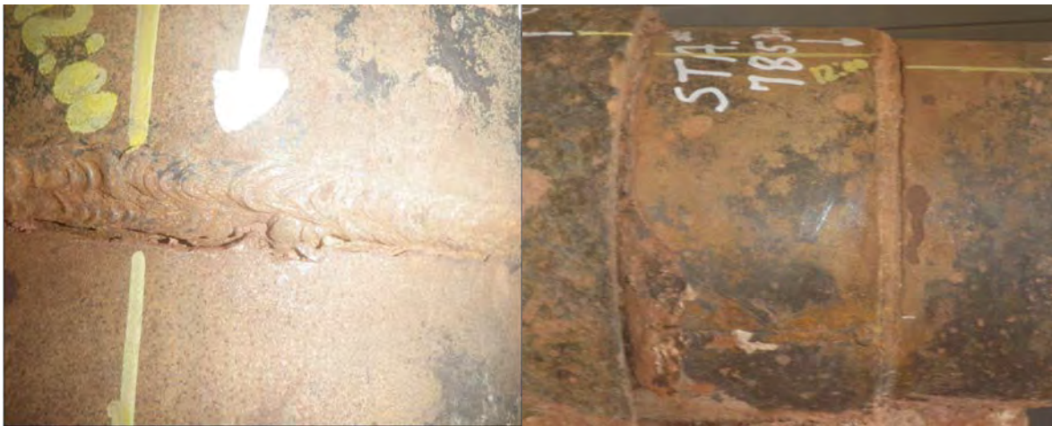
Photos 4 and 5 – Showing the failure and the location of the failure
