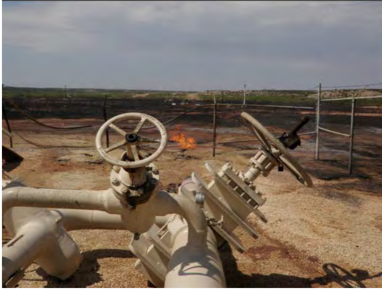
Photo 1 – Facing upstream on line that failed
