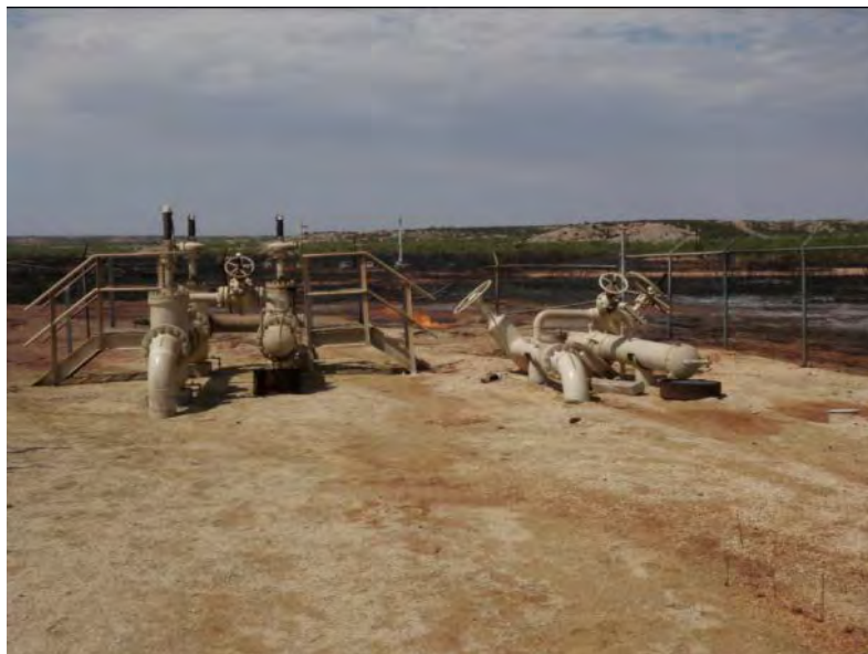
Photo 2 – Pig trap area facing upstream
