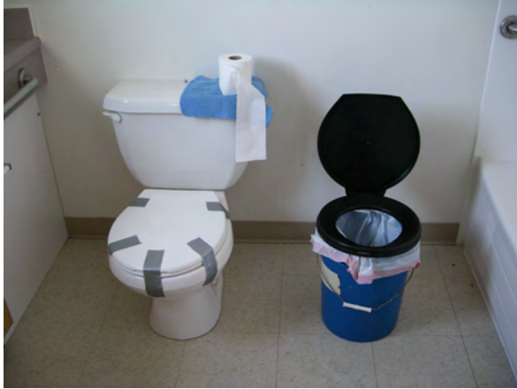
Honey-bucket, above, at Stebbins Elder Housing Center. Flush toilet, left, remains sealed and unused years after construction.
