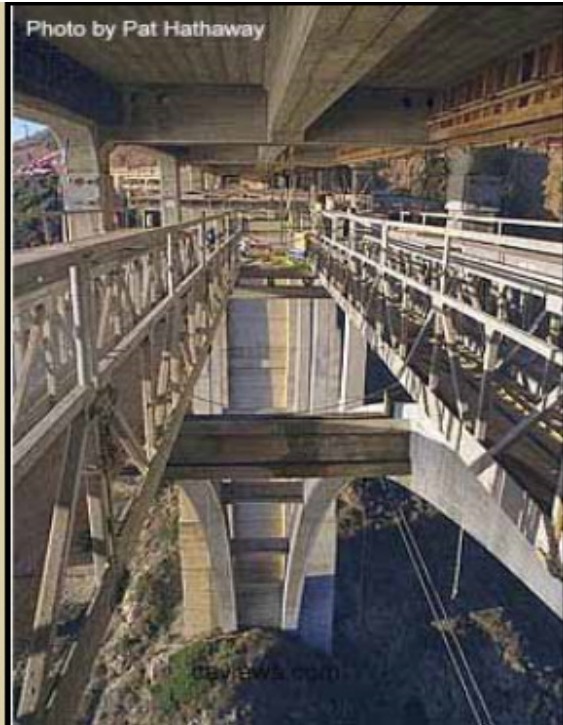
Figure 14: View from under the deck on a temporary platform during the retrofit
