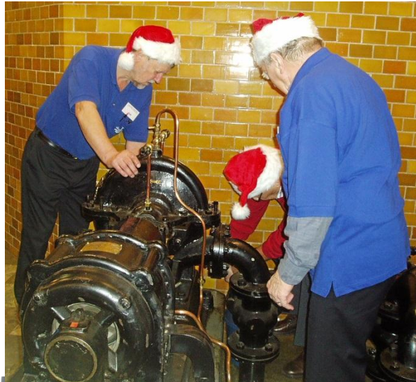
Alexander members preparing for the cooling pump to be started for a Christmas Eve transmission.
