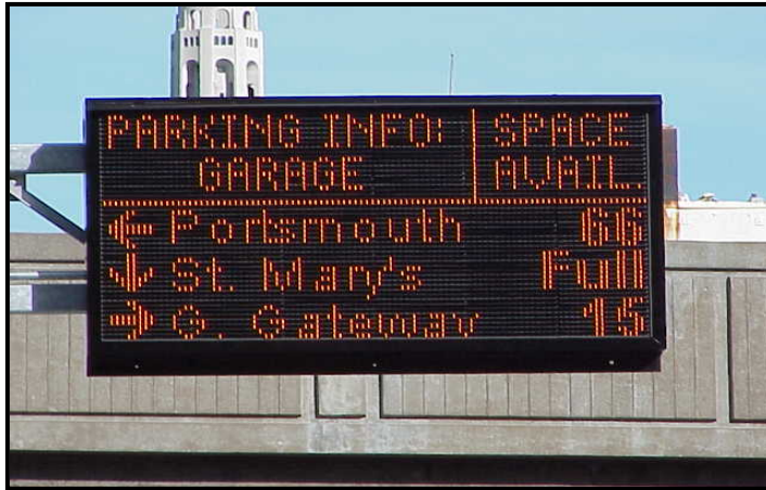
Figure 1-8. Variable Message Signs Will Guide Drivers to Available Parking in San Francisco
