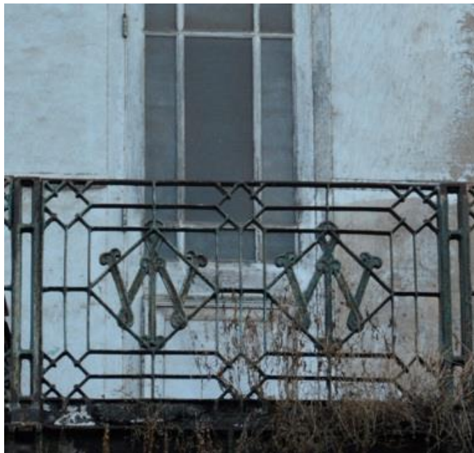
FIGURE 3.2 & 3.3. (Above) The Esplanade Hotel, Fort. (Below) The balconies of The Esplanade Hotel were decorated with the monogram 'W' (for Watson) and indicate the ways the proprietor inserted his identity into the Hotel space and structure.
