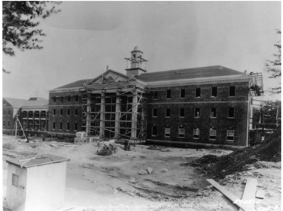
► The new nurses quarters, Delano Hall, under construction on April 8, 1931. The Hall had 196 bedrooms for nurses assigned to the hospital. It had sunporches, music rooms, reception rooms, and a ballroom. It was named for Jane Delano, the second superintendent of the Army Nurse Corps. Source: National Archives and Records Administration, SC 590550
