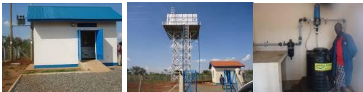
L-R: 60kVA generator in generator house and 50kVA transformer; 200m 3 steel reservoir tank; Chlorine dosing equipment in Pajule Town Board
