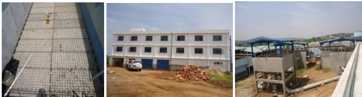
L-R: New backwash nozzles installed in the slow sand filter; Offices and Chemical building; Distribution and reaction chamber at Gaba II water treatment plant
