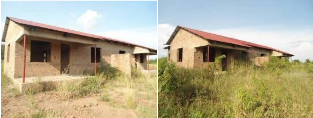
Two semi-detached houses left incomplete at Engineer Kauliza Kasadha Technical Institute, Bugiri District
