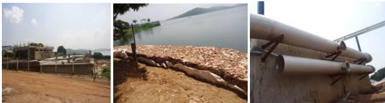
Left: New reservoir and pumping station; Center: Gabions on the lake shores; Right: Sludge recirculation pipes at Ggaba I water treatment plant
