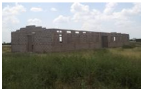
Abandoned dormitory at Lolachat P/S, Nakapiripit district
