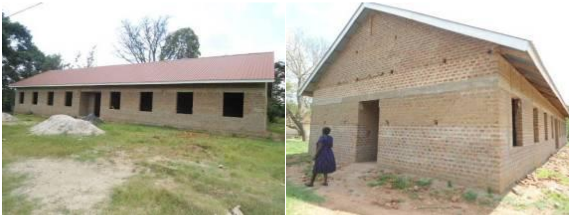
The two dormitory blocks (one for boys and one for girls) constructed at Kaliro PTC
