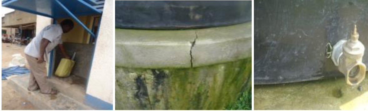
L-R: Functional public kiosk in Nyeihanga town; Cracked concrete tank base in Kashozi sub-county; leaking joint on the Kashozi tank
