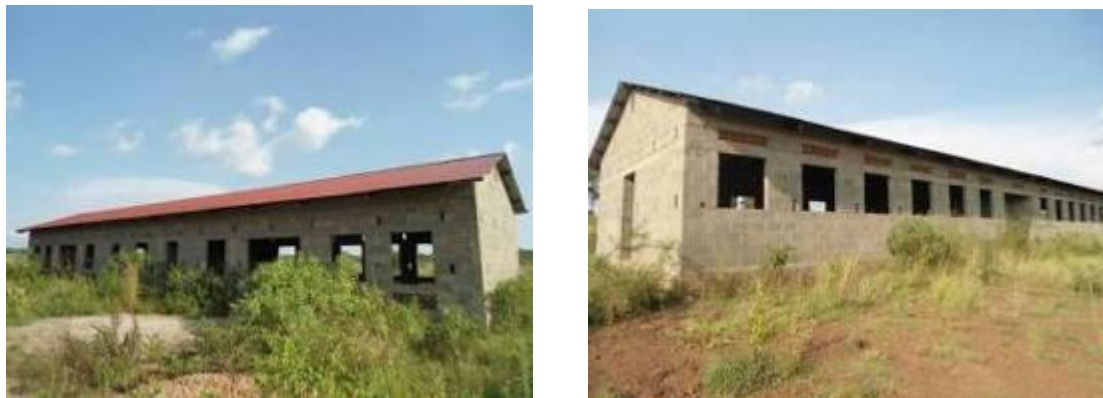
Two workshop blocks left incomplete at Engineer Kauliza Kasadha Technical Institute – Bugiri District
