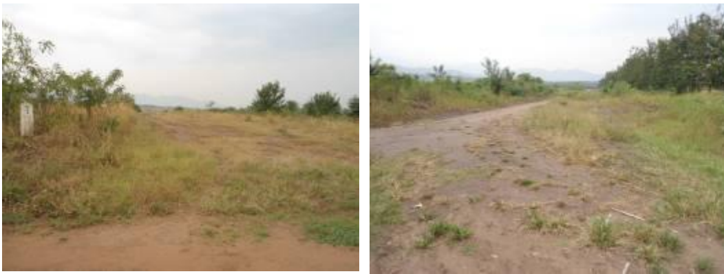
Incomplete and abandoned road workss in Kasese Industrial Park
