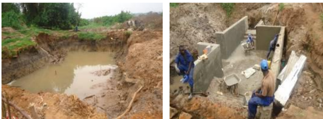
L-R: Excavation of the reservoir and construction of the community well at Kiboga Hospital
