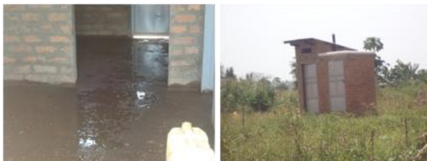
Left: newly cemented floor in house of beneficiary; middle: bathroom facilities in Zone B1, Kiryandongo district
