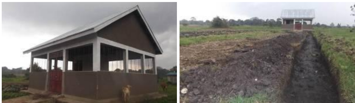
L-R: The completed slaughter slab, and the excavated foundation trench in preparation for construction of an access road to the facility at Namaira Trading center, Kamuli District
