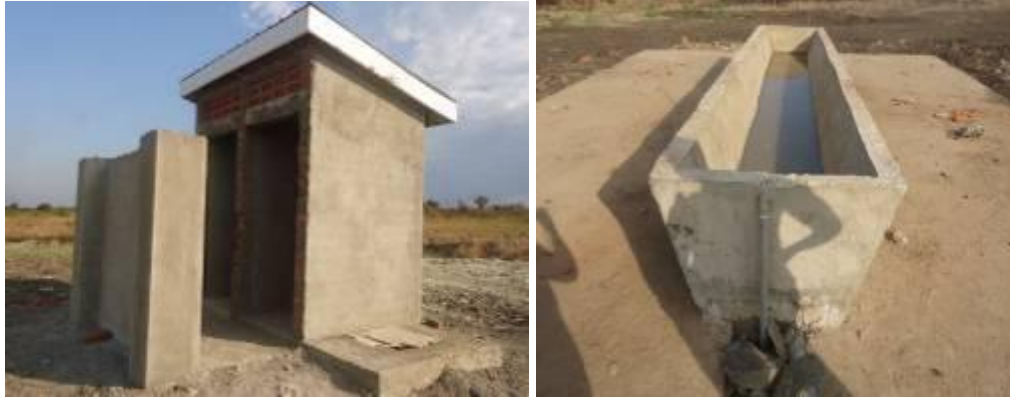
L-R: VIP toilet; Cattle trough in Panyango sub-county
