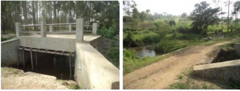
L-R: Side view of bridge and the temporary road used by community in Yerya village, Kabarole district
