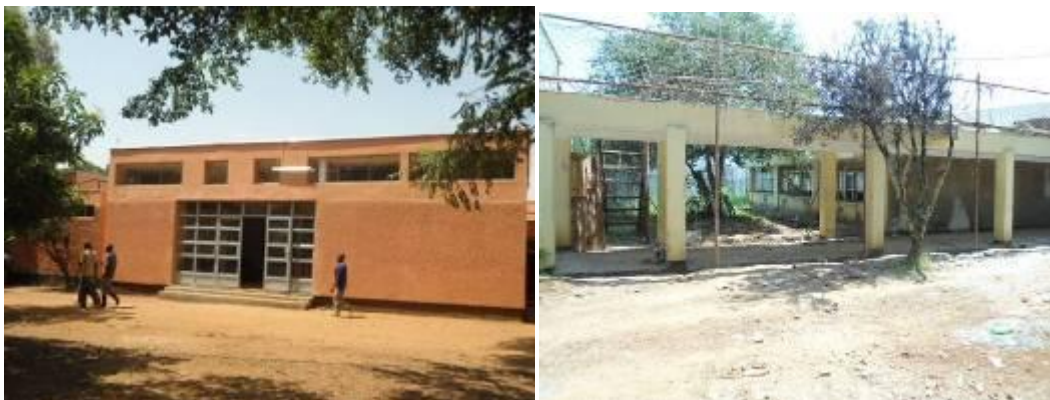
Left: Block 'Y' renovated, Right: Renovation of block 'X' on going at Kaliro NTC
