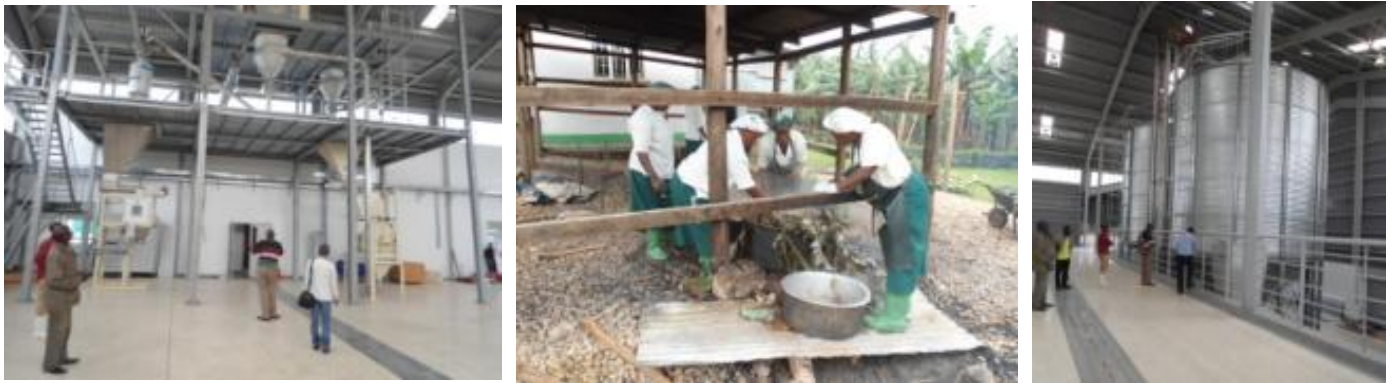
L-R: Partially installed Hammer mill, ladies preparing instant Tooke and installed Silos at Nyaruzinga-Bushenyi
