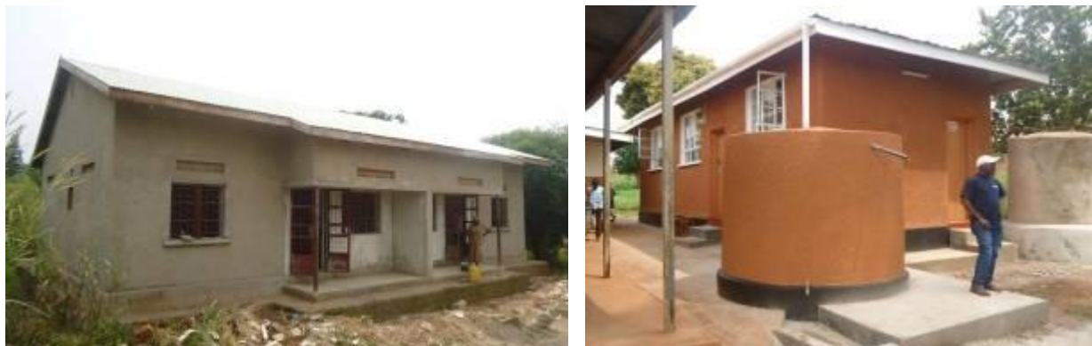
L-R: Semidetached staff house under construction and rehabilitated general ward at Ikooba HCIII, Masindi district
