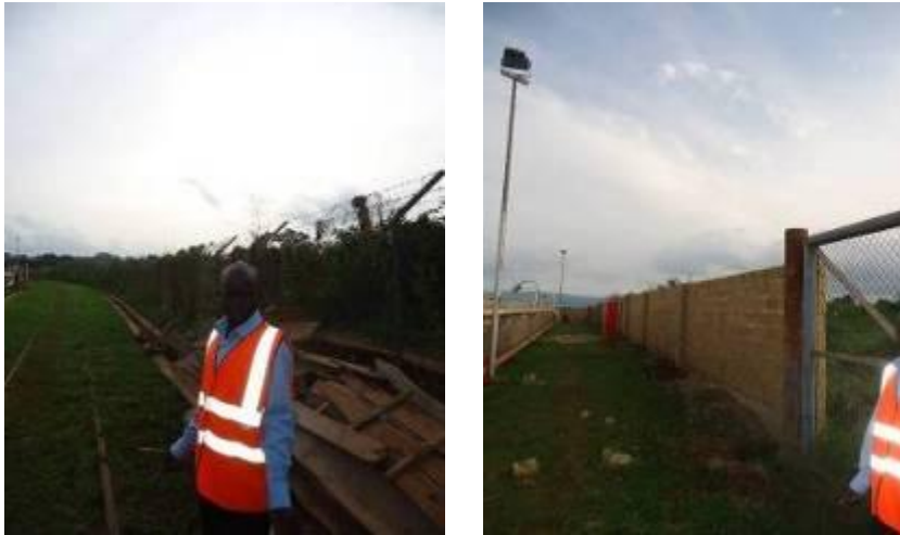
L-R: Completed and incomplete section of the wall fence at the Jinja storage tanks
