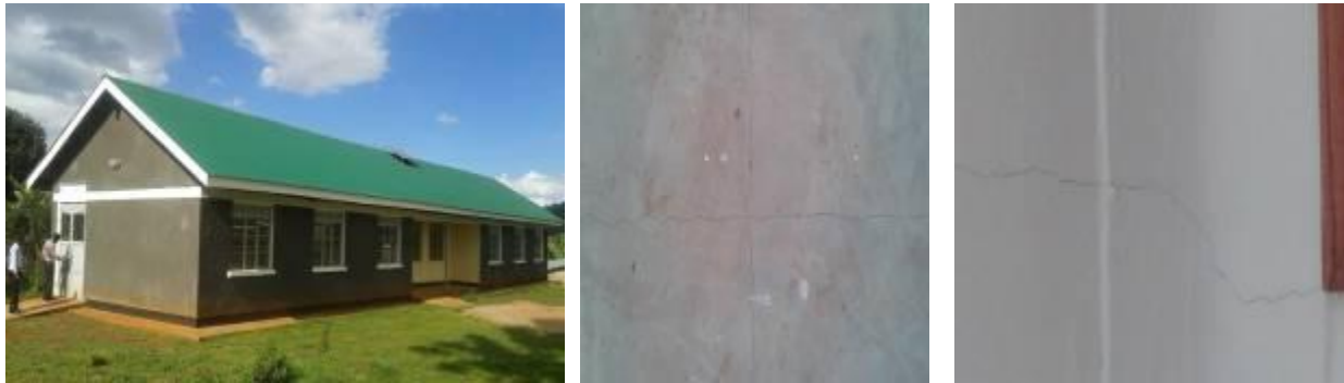
L-R: Maternity ward and the defects on the floor and ceiling at Kabeywa HCIII, Kapchorwa district
