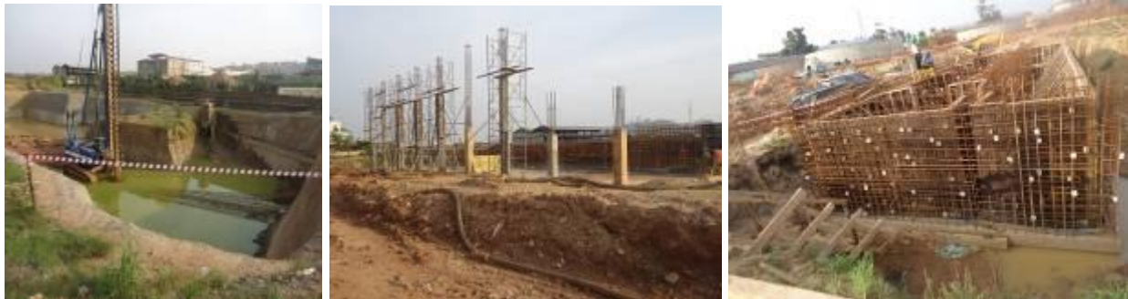
L-R: Pile foundation excavation for inlet pumping station; Columns for the pretreatment structure/chemical house; and Reinforcement bars for the trickling filter pumping station walls at Bugolobi, Kampala district
