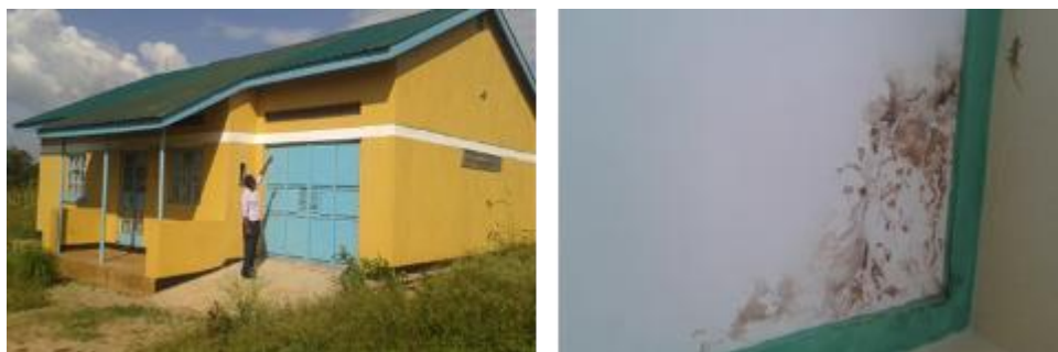
L-R: Renovated Doctor's house and a leaking ceiling at Nankoma HCIV, Bugiri district
