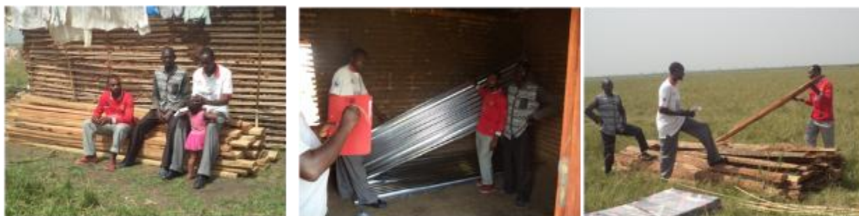
Left: Timber purchased by the group; Middle: Iron sheets for roofing; Right: Pieces of wood for construction in Kirunga village sub-county, Ntoroko district
