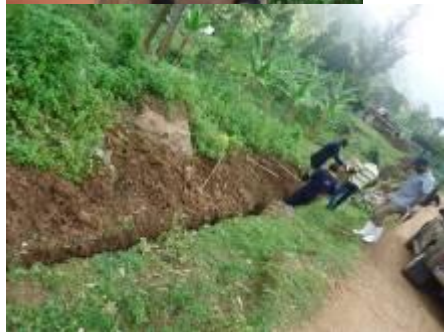
L-R: Cracked verandah of water office; Stud columns for reservoir tanks; Trenching for distribution pipes, Bududa district
