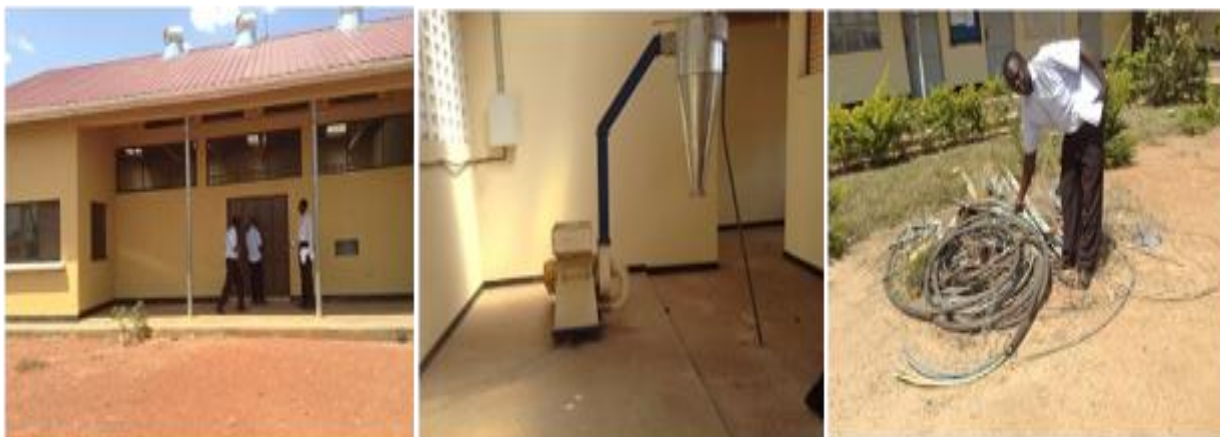
Left: Non-functional APF, Middle: Incomplete rice mill installation abandoned; Electrical items abandoned by the contractor since August, 2015 at barr-subcounty in Lira district
