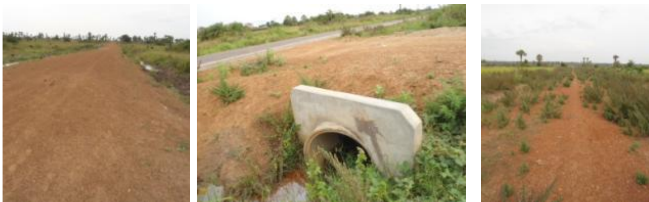
L-R: An opened gravel road, a cross culvert joining to Temele road and an overgrown opened road in Soroti Park. The new roads do not have traffic and are not in use
