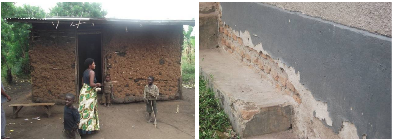
Left: A PAP in Kitcwamba Sub County, Kasese district cannot make developments on the house and yet payment has delayed to enable her relocate. Right: Shoddy resettlement house in Rwimi Sub county, Kabarole district
