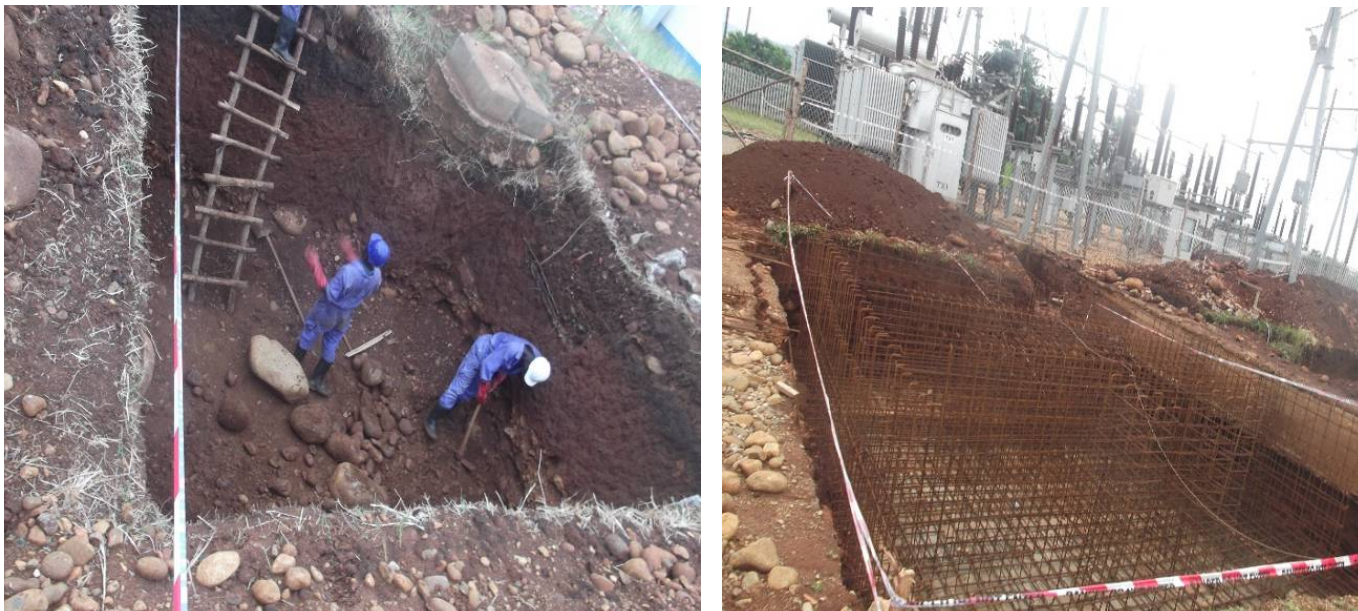
Left: Manual Excavations of hard rock Right: Preparatory works for concrete casting on Nkenda substation in Kasese district
