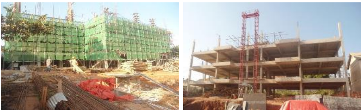
Left: Ongoing works on the main hospital block, Right: staff house at Kiruddu General Hospital
