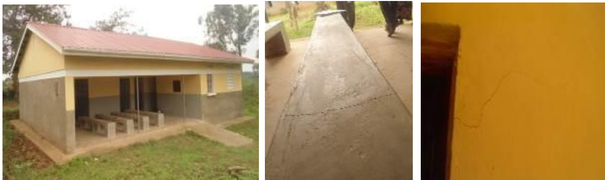
Left: Completed OPD, cracked patient bench (middle) and cracked wall in the new OPD at Kashongi HCIII (Right)
