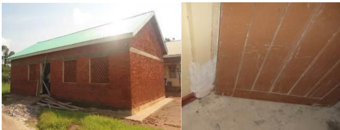
Left: Renovation works of the OPD and Right is the old door frame filled with FILA instead of replacement at Budima HCIII in Jinja District
