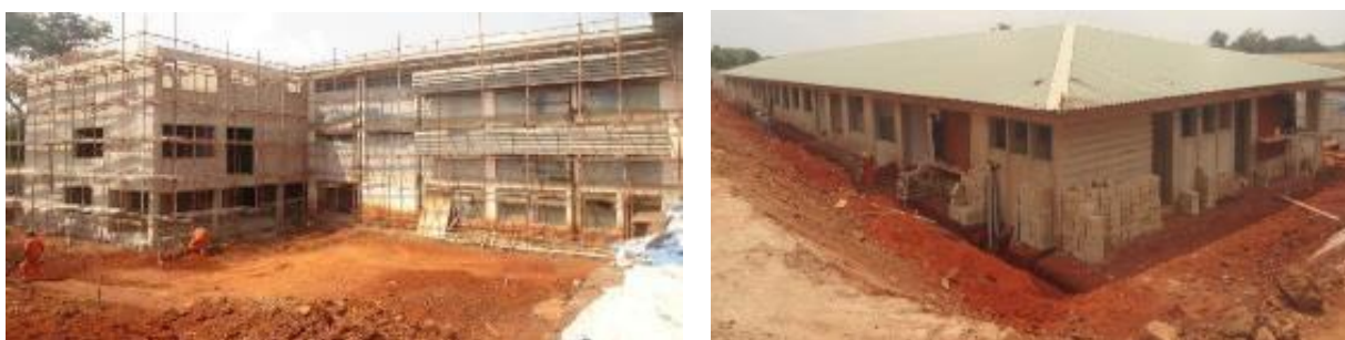
Left: Ongoing expansion works on the existing T-block. Right: new OPD under construction at Nakaseke Hospital
