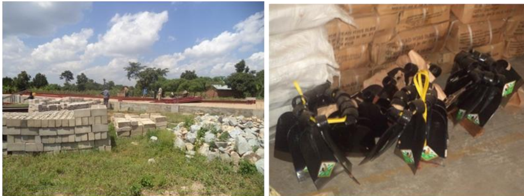
Left: Workers assembling metallic poles on foundation of Butaleja produce store at Butaleja Town Council; right: Hand hoes purchased using relocated funds for construction of Chiefs' complex kept at OPM central stores in Kampala
