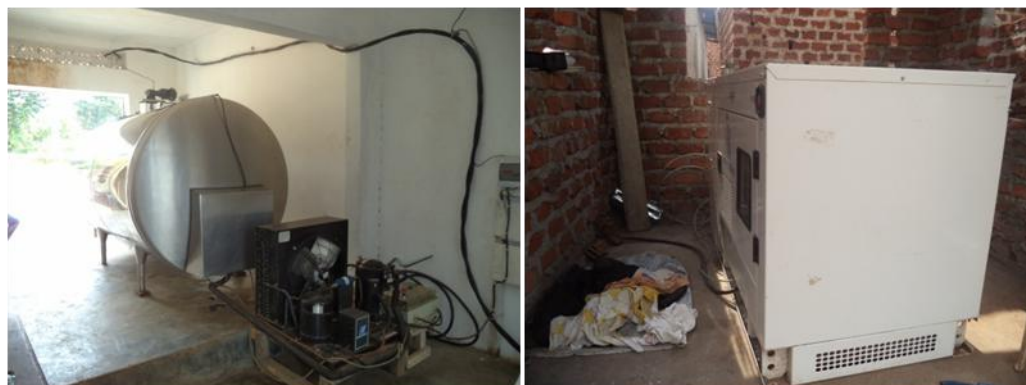
Left: Milk cooler; right: Generator purchased by the project in Bukomero Town council, Kiboga District
